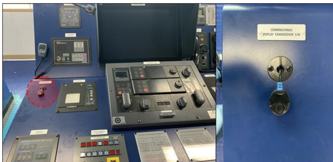
Figure 4: Hardware selector for switching between conning display and HiNAS2.0 display at the centre console
