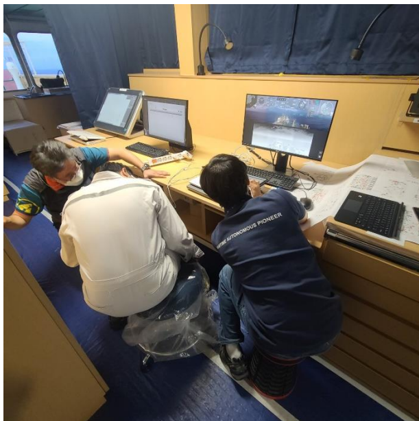
Figure 5: HiNAS2.0 monitor on the chart table (checking the installation is well completed)
